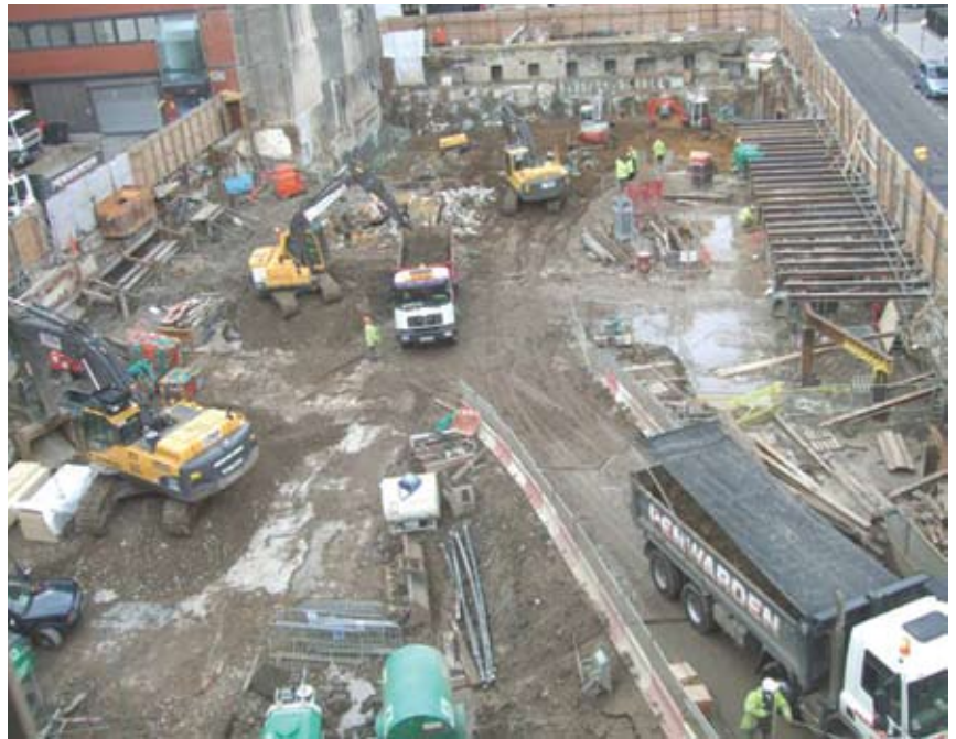
Building work starting on the site of the new Cancer Centre on Huntley Street
